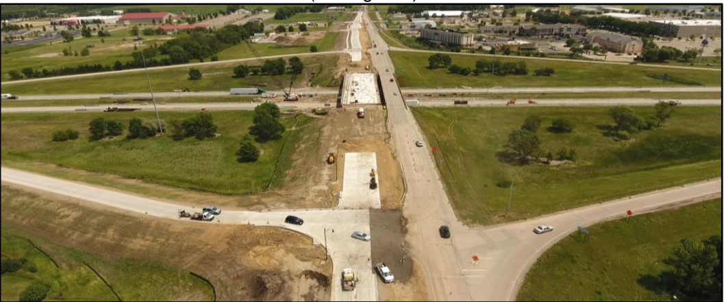
Project Photo: Bridge & adjoining pavement work @ the new I-29 bridge. (looking east)
