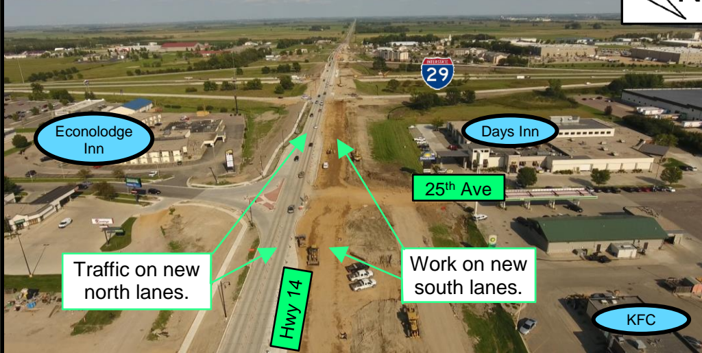
Project Photo: Overview of work on south lanes of project (looking east)
